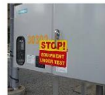
Use of “STOP - Equipment Under Test” Magnet
