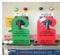
Use of Flagging Hangers “Testing in Progress” and “Do Not Operate”
